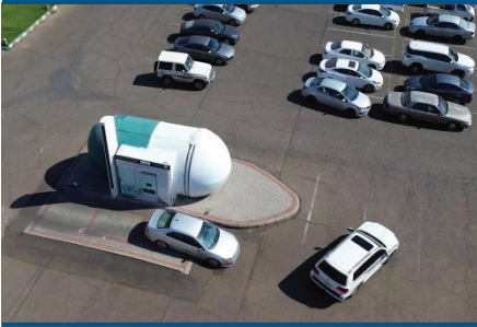
Parking lot and outpatient lobby congestion are eased since 25% of the pharmacy's total daily orders are picked up at RoboWall.
